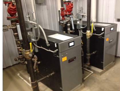
New High-Efficiency Boilers 2012
